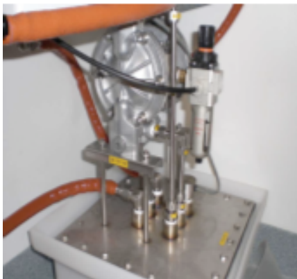
Under bench Waste Transfer Station
